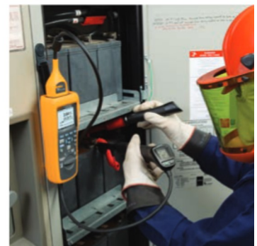
Measure impedance with the Fluke BT521 Battery Analyzer.
