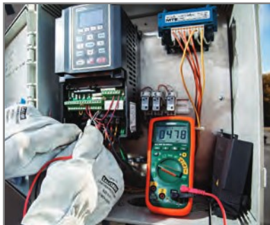
Low Pass Filter (LPF) ensures accurate AC Voltage measurements on a variable frequency drive.
